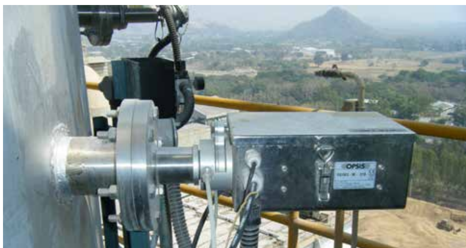
OPSIS' products are used in waste treatment plants to monitor stack emissions and for process control.
